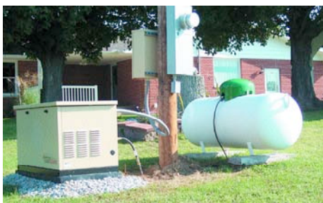
Installation of 100 of these generators at homes and small businesses will help the Shelby Electric Cooperative during peak-demand periods and during power outages.
