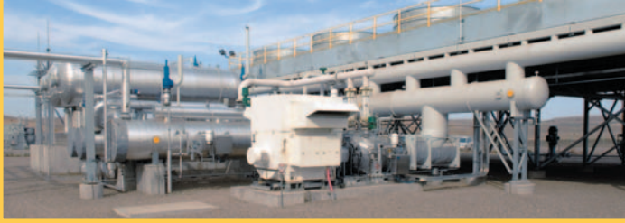
Heat-recovery units on Basin's Northern Border natural gas pipeline recover waste heat generated by gas turbine-driven pumps that move gas along the pipeline. The heat is then used to generate electrical power.
