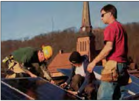
Looking for a few good roofs – the Clean Energy Cooperative of Northern Pennsylvania is gearing up for rooftop installations of solar panels.
