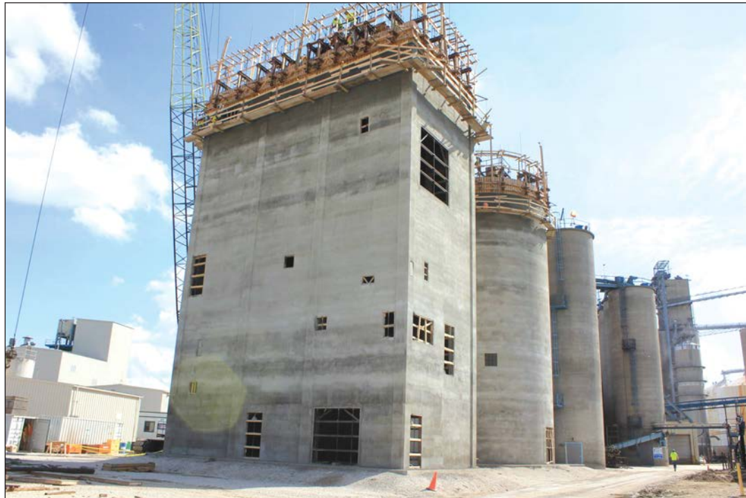
Cement silos are part of an expansion at West Central's SoyPlus plant. As of April 1, West Central, Ralston, Iowa, and Farmers Cooperative Co., Ames, Iowa, are merging. Photo courtesy West Central.
