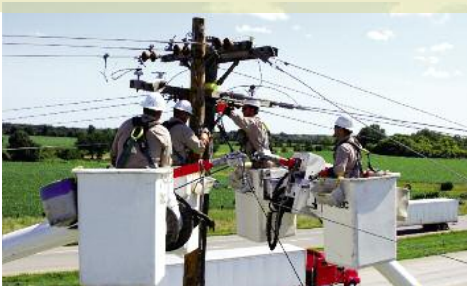
A crew from Callaway Electric Cooperative (CEC) works on power lines in its rural Missouri service territory. Photo courtesy CEC
