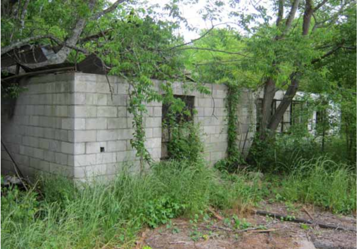
Figure 108. A deteriorating cinderblock farm structure in the easternmost survey area. View northeast.
