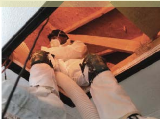
Blowing insulation into an attic can have a major, beneficial impact on a member's heating and cooling bills. Photo courtesy Roanoke Electric Membership Corporation
