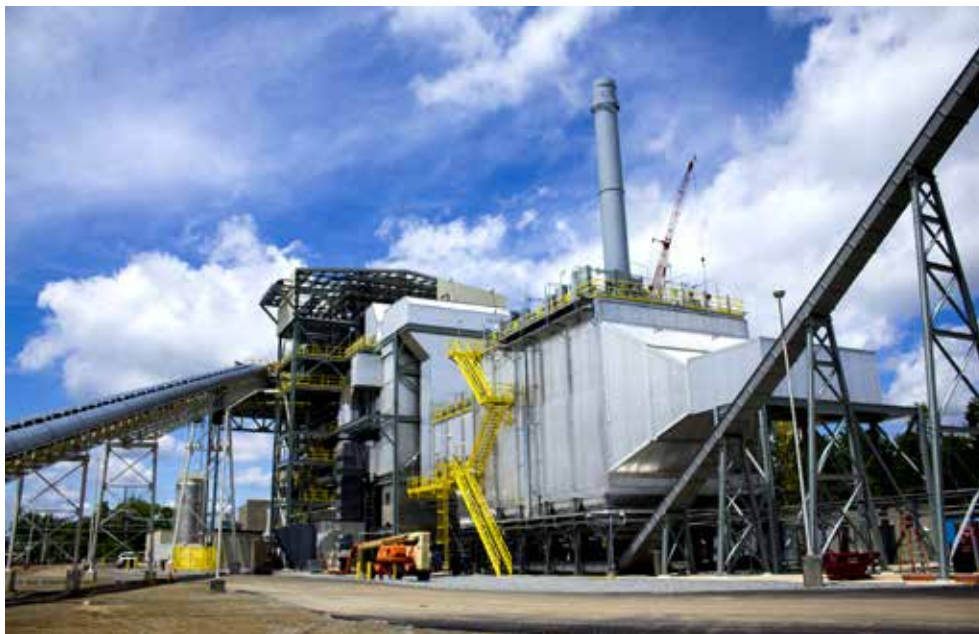
This biomass plant in Halifax County, Va., burns wood waste leftover from logging, generating enough power to light up 16,000 homes. Photos courtesy Northern Virginia Electric Cooperative (NOVEC).
