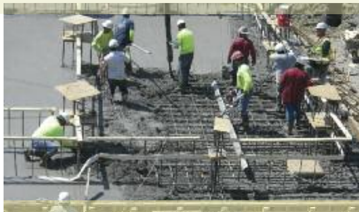
Construction work progresses on New Vision Cooperative's Magnolia feed mill project, a $16 million elevator/feed mill slated to begin operation in June 2013. It will create 12 jobs in its first year of operation. Photo courtesy New Vision Cooperative
