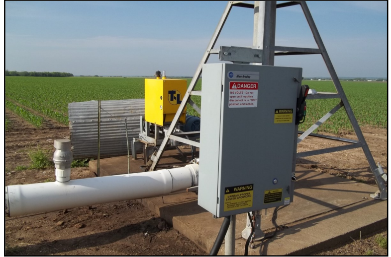
Electric motorized Pivot pump for agricultural producers
