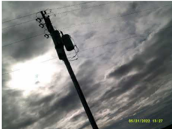
Photo #7 View of three-pole mounted transformers next to well house.
