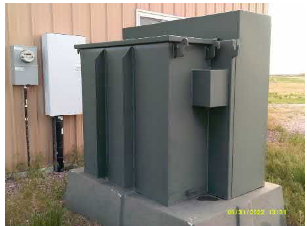
Photo #10 View of pad mounted transformer next to well house looking east.
