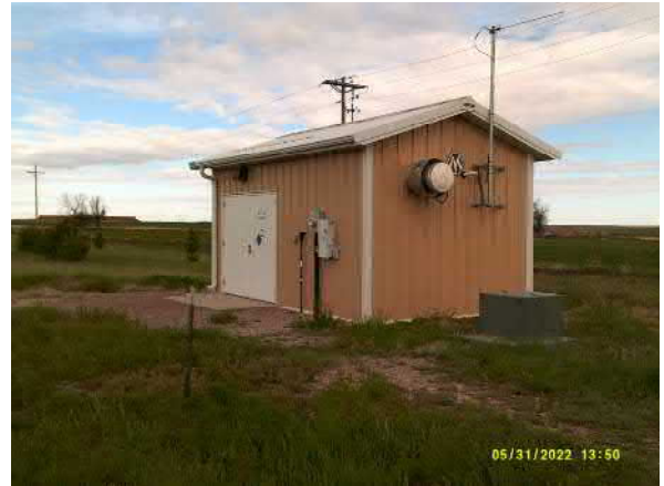
Photo #20 View of pad mounted transformer on northeast corner of site.
