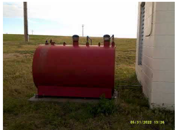
Photo #4 View of red above-ground storage tank next to well house (#2) on site.
