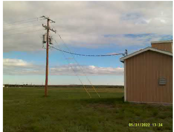
Photo #2 View of three pole-mounted transformers just west of the northeast well house.
