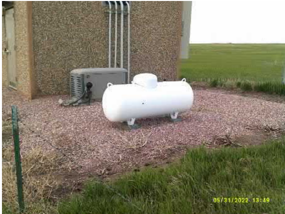
Photo #19 View of small aboveground storage tank next to electrical building on northeast corner of site.
