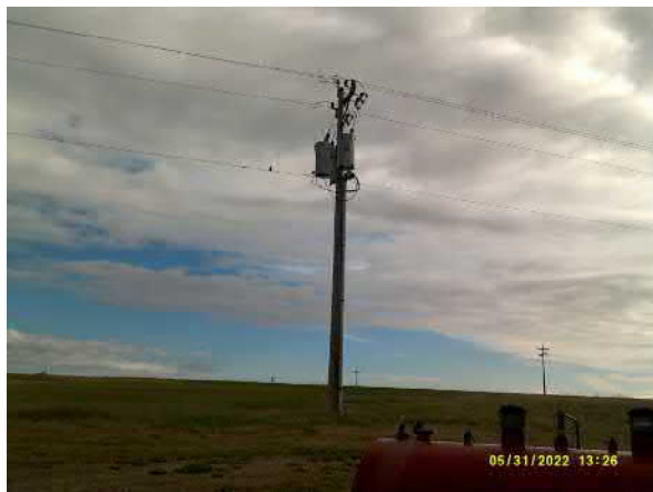
Photo #5 View of three pole-mounted transformers next to well house.
