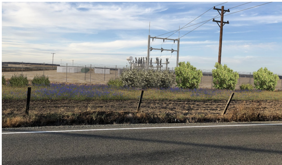
Figure 3.7-4. KOP 3 Dillard Road near Project entrance, facing west; approximately 200 feet to the generation tie line backed by battery energy storage and solar panels
