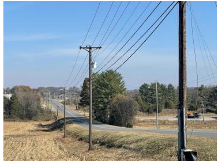
Photo 10 View of pole-mounted transformer facing northeast
