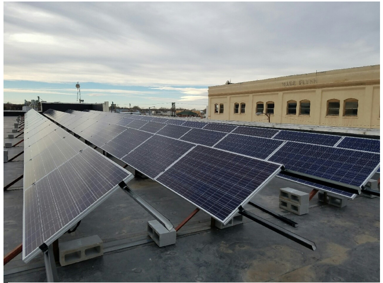
Rooftop Solar Unit Located on Top of the Bluffs Business Center Building.
