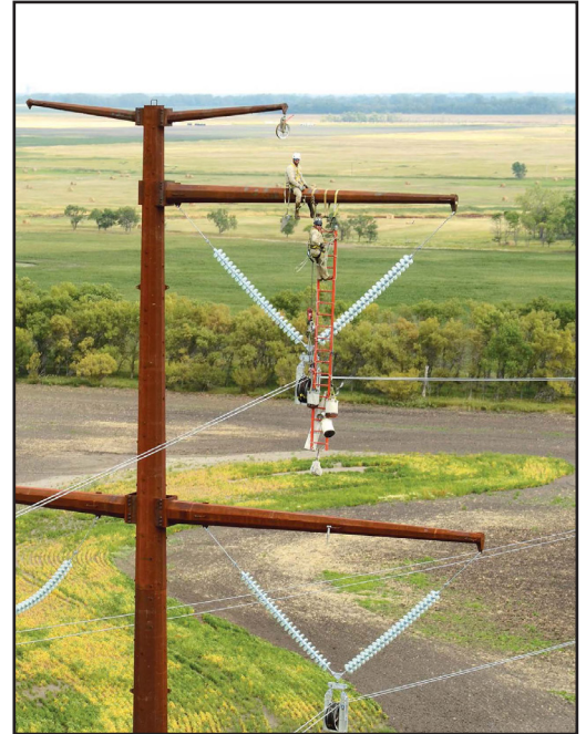
Crews clip in a CFG line segment. Clipping is removing the wire from the pulling dolly and attaching it to the insulator string. Workers use safety harnesses and ladders to do this challenging job. Photo Courtesy of Minnkota Power Co-op.
