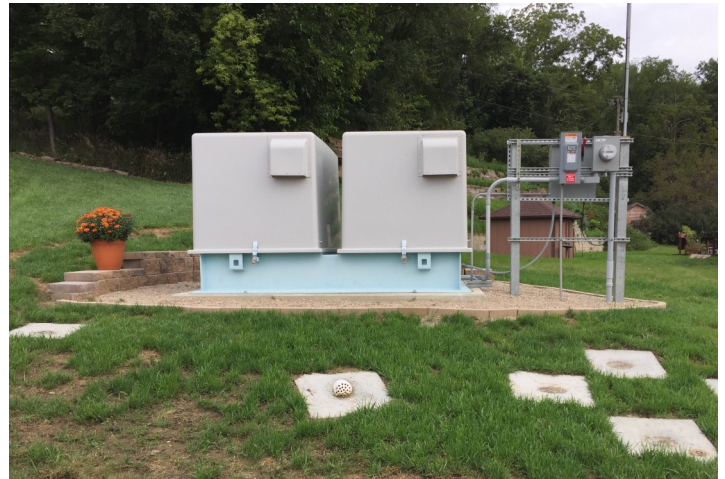
A booster station was installed to give better water pressure to residents in town, especially along Ry Miller Street.
