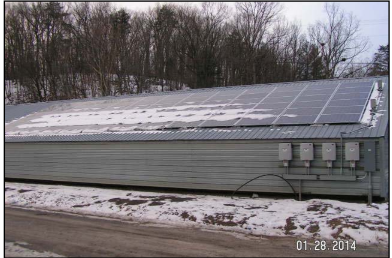
Malcolm Farms Operational Solar Panels
